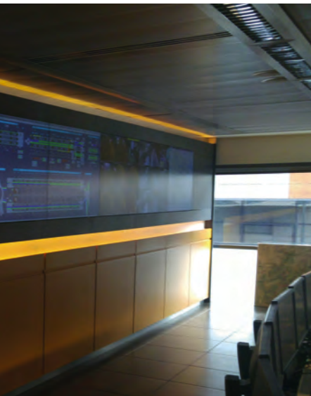
(Above and left) Rear projection LED screens at Cenatra traffic control center
