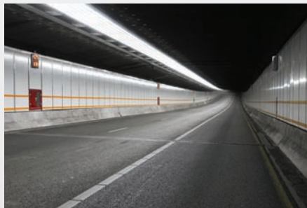
Linear LED lighting provides a much improved and safer driving experience for tunnel users
